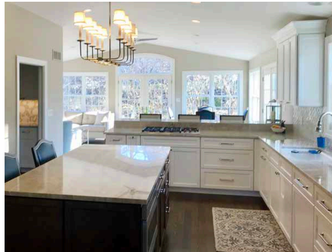
Kitchen remodel with floor, cabinets, stone countertops, fixtures, appliances, lighting, and more!
