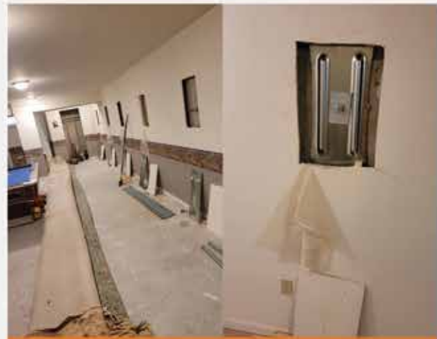
BOWED WALL REPAIR
