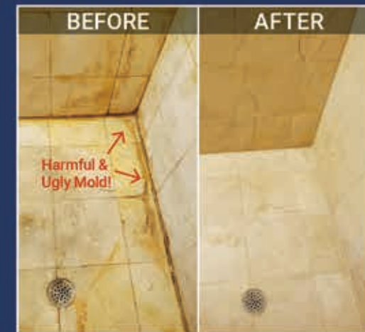
Shower Tile Mold Remediation
