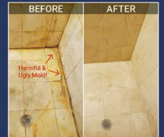
Shower Tile Mold Remediation
